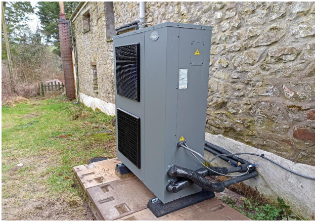
New Air Source Heat Pump
