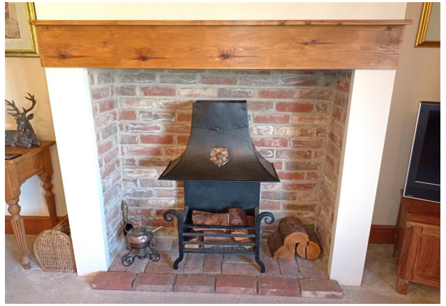
Feature Fireplace (no flue)
