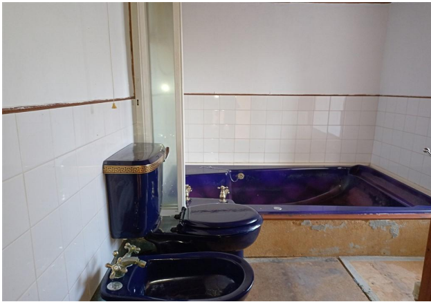
Master Ensuite Needing Refurbishment
