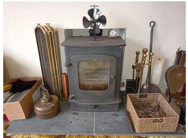
Woodburner In Lounge
