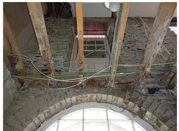
Rotten Joists On 1st Floor
