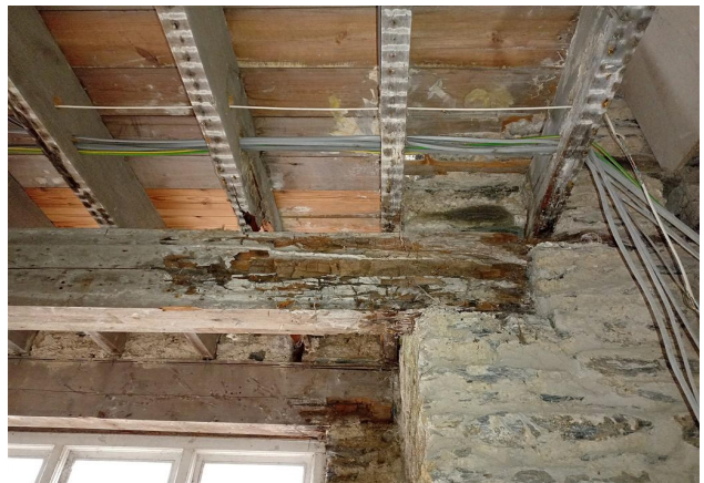
Two Rotten Structural Beams
